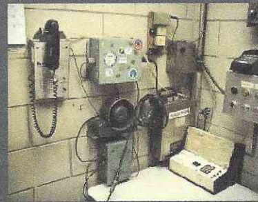
Example of a communication station for dispatcher
