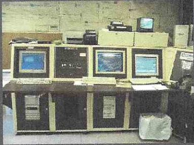
Example of a mine wide monitoring control room
